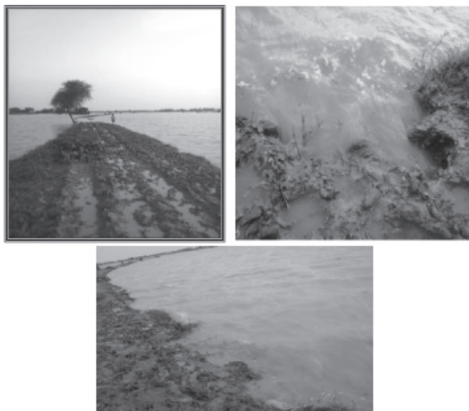
A view of Road damage due to severe flood
